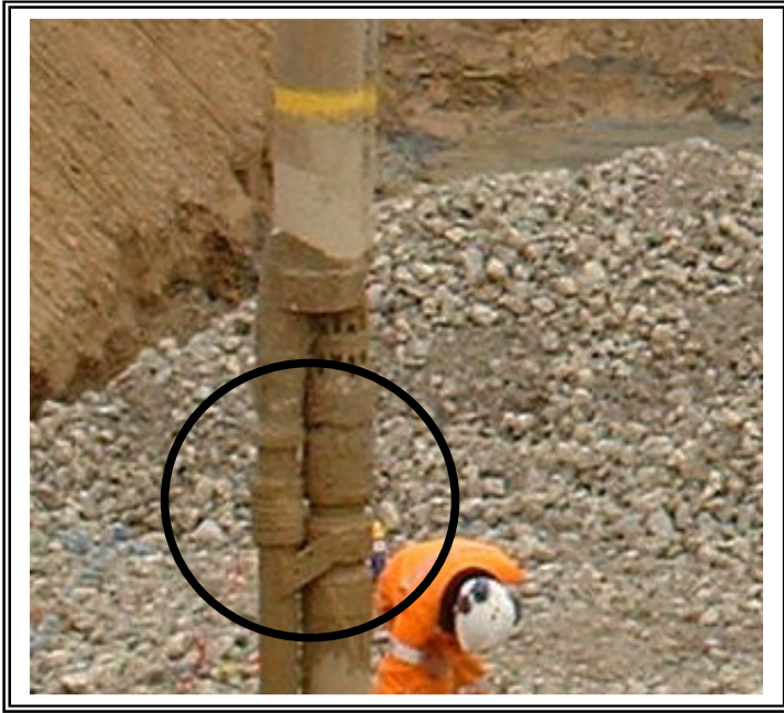
Figure (5) highlights the location of the rubber isolator; the yellow horizontal marking is an indication for the reader to locate the isolator position in figure (3) pictured above.
